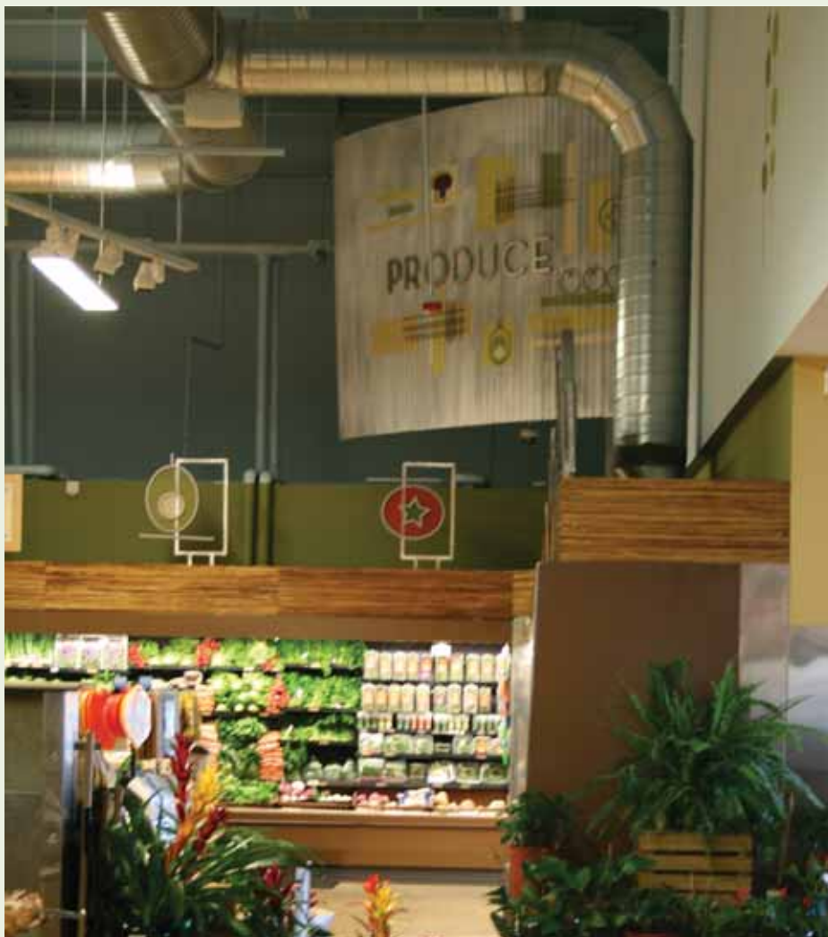
Exposed produce refrigeration ducts efficiently re-circulate the heat, which is then used to warm the building's water systems.
